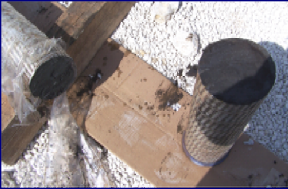
CP720 FILTER PLUGGED WITH SOLIDS
